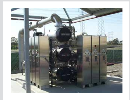
The TrojanUVPhox™ installed at the Leo J. Vander Lans Water Treatment Facility.
